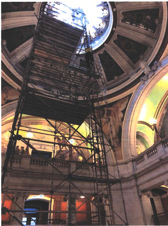
Figure 4. Initially, ceiling panels were accessed with a mobile scaffold tower. (Photo by EverGreene, June 2020)
