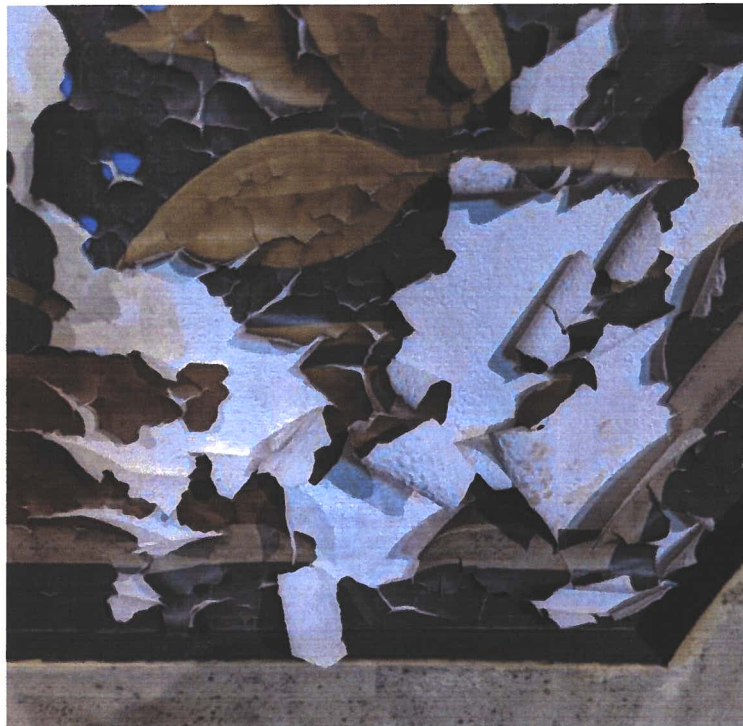
Figure 7. Detail of severe paint detachment and curling at "Capricorn" panel. (Photo by EverGreene, July 2020)
