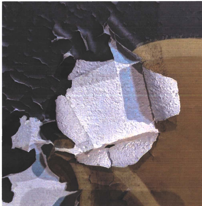
Figure 8. Detail of plaster deterioration (efflorescence and chalking) at "Capricorn" panel. (Photo by EverGreene, July 2020)
