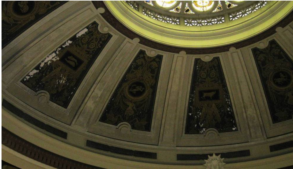
Flaking and loss at the dome ceiling
