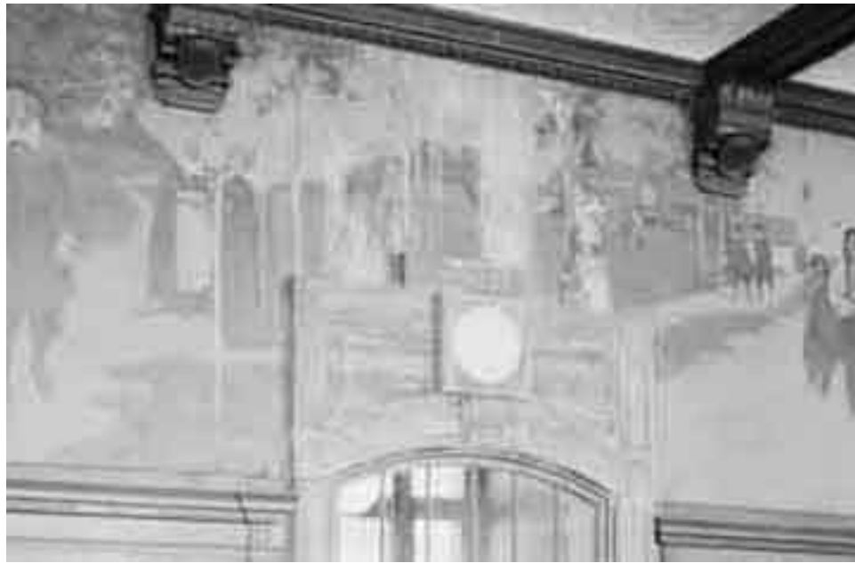
Archival photograph (detail) of water damage
