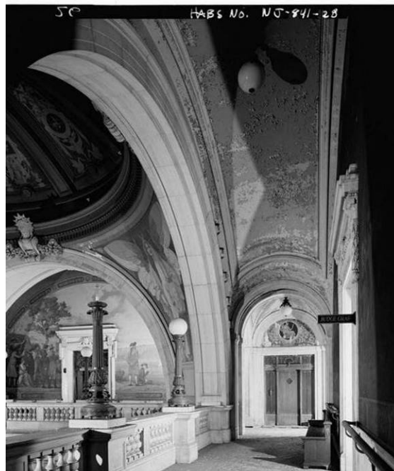
Vast areas of water damage and flaking paint, as captured in the above HABS photograph, would have necessitated the scraping and skimming
