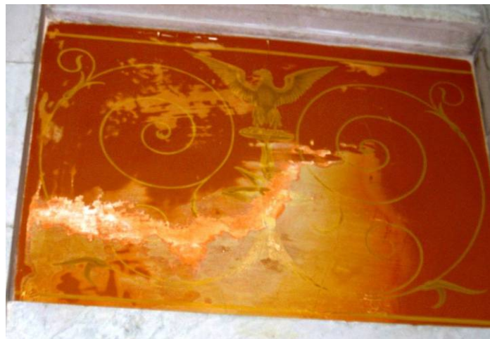
Water damage, staining and efflorescence at the second floor frieze (SE corner)
